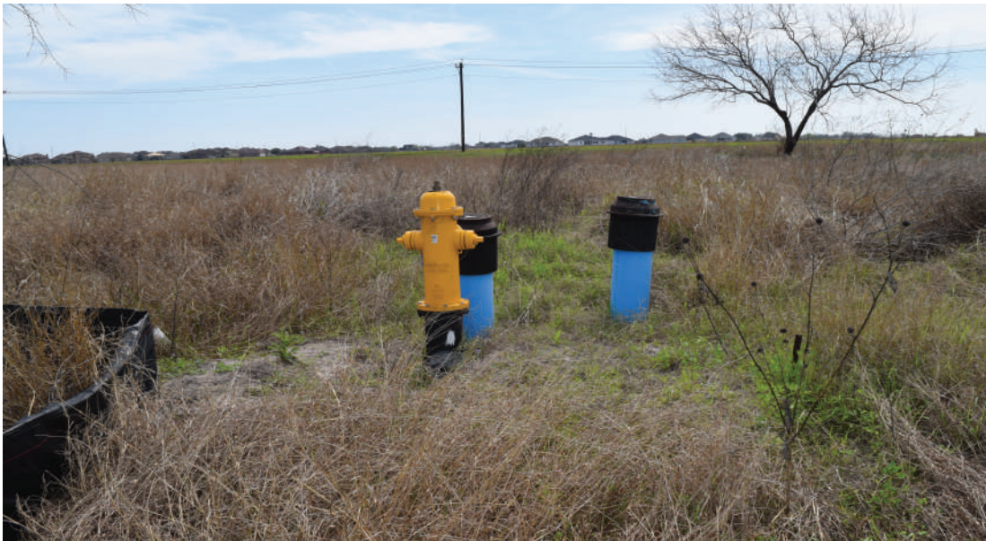
Southerly view of the property, with fire hydrant and sewer line stubs
