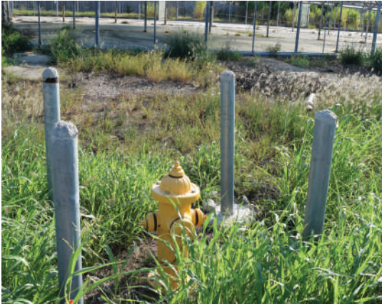
One of two fire hydrants on property
